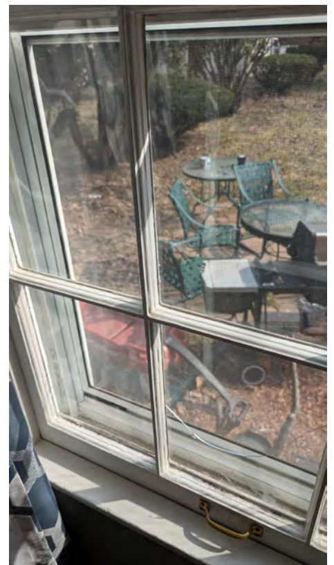
8. interior detail view. notice cracked pane and moisture
