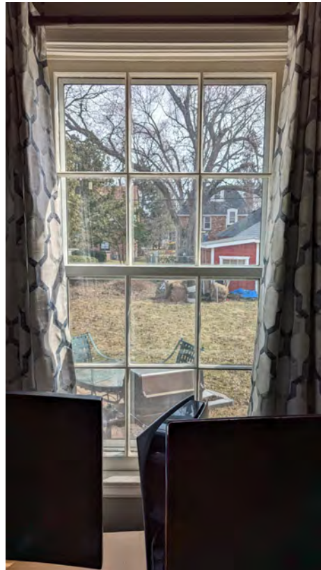
8. interior view also pools moisture
