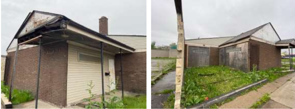
Photos of the 7569 Tireman property owned by Mr. Cooper
