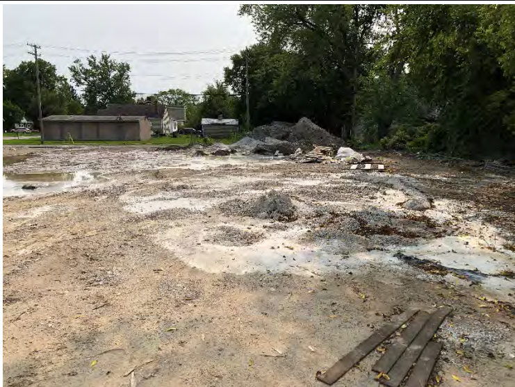
Photo 2. View of concrete washout piles and the crushed asphalt pile in the background
