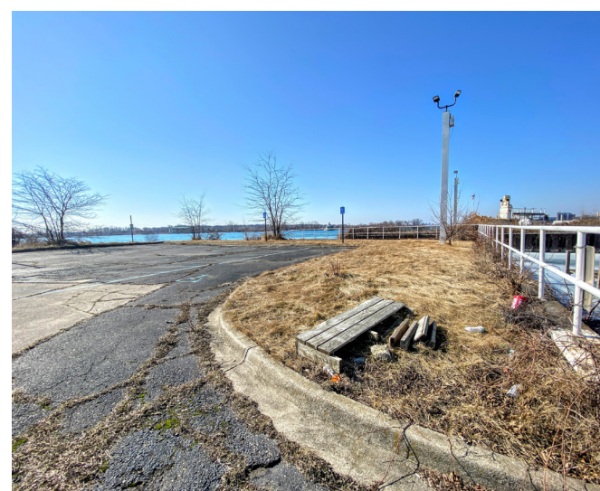
Parking lot and curbs are in poor condition
