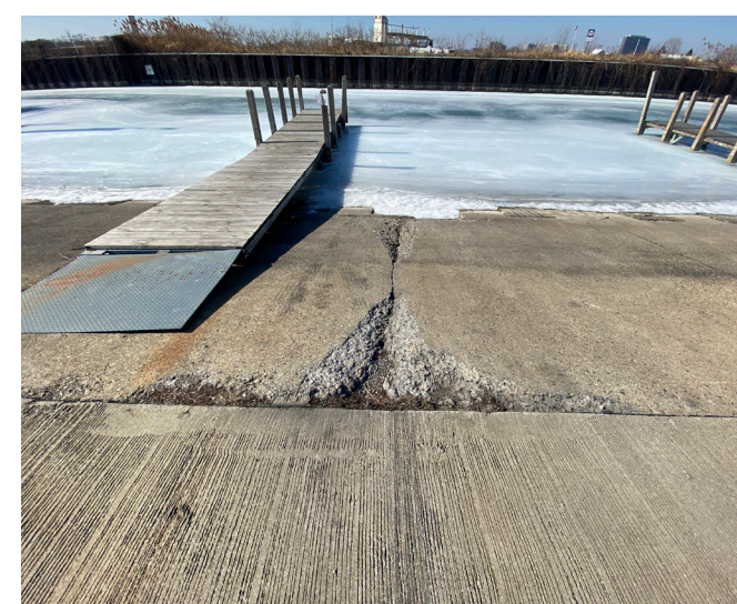
Concrete pad at the launch showing large potholes
