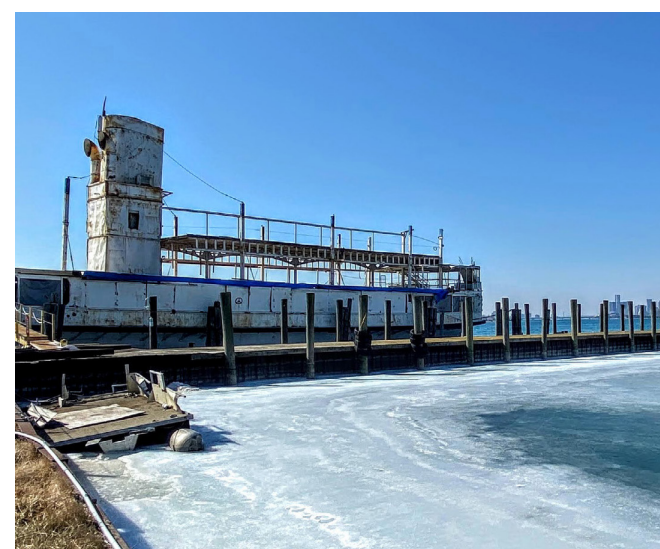
The large boat pier at the south entrance has wooden decking in need of replacement
