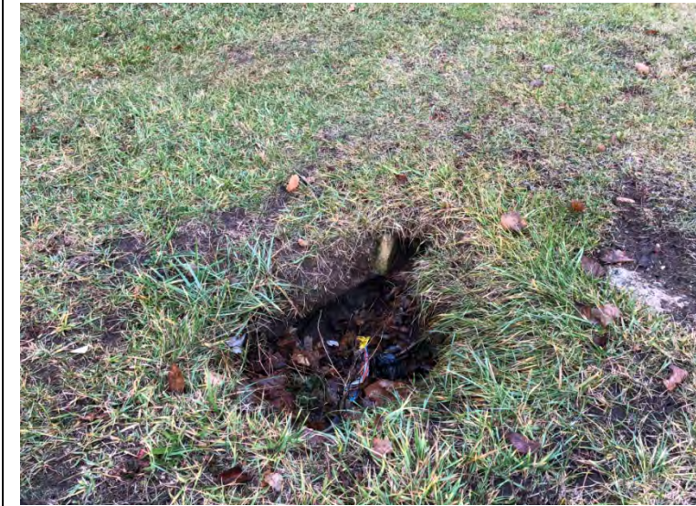
Photo 13. Another example of the ground depressions
