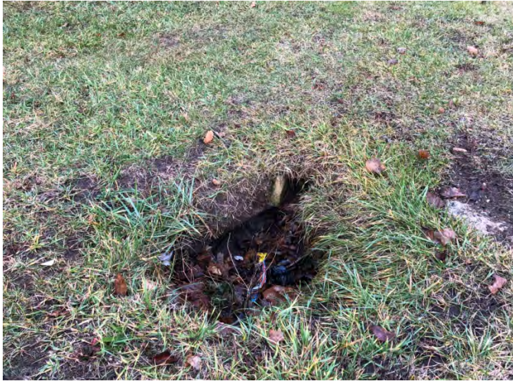
Photo 13. Another example of the ground depressions
