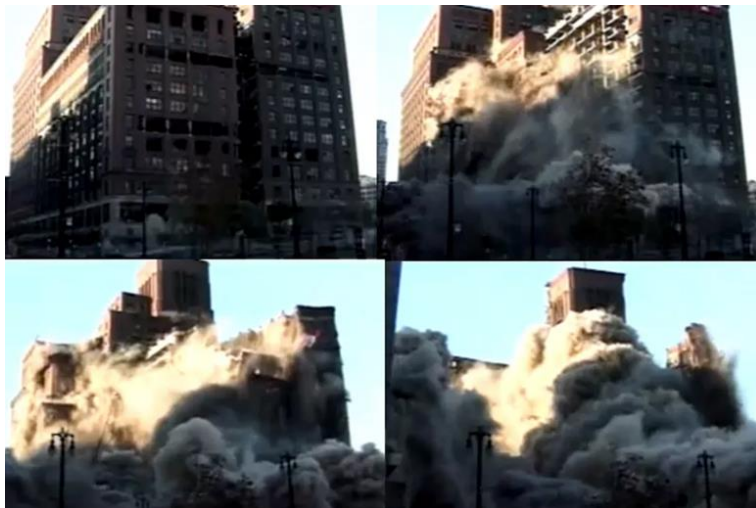
The controlled demolition of the Hudson's Department store at 5:45 p.m. on Oct. 24, 1998 11
