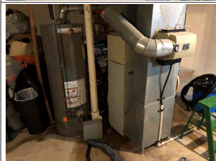
Photo 11. Example water heater and furnace
