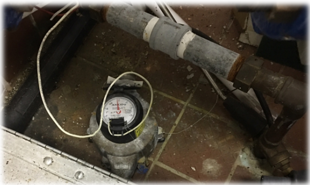
Straight-piping investigation by the Fraud Unit
