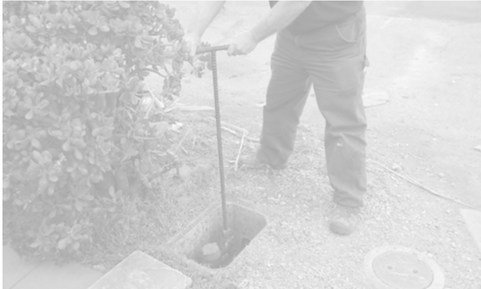
Water theft with unauthorized turn-on
