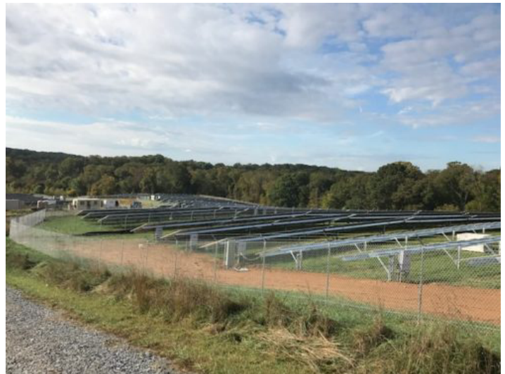
Figure 15: Nixon Farm solar garden - Power52 solar farm project, BGEC Community Pilot Site 20
