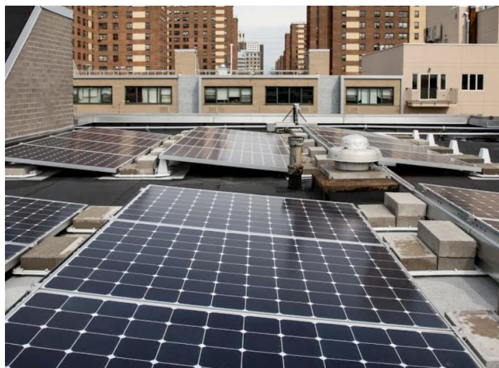
Figure 16 Rooftop arrays of Marcus Garvey Apartments Microgrid, Brooklyn, New York 21
