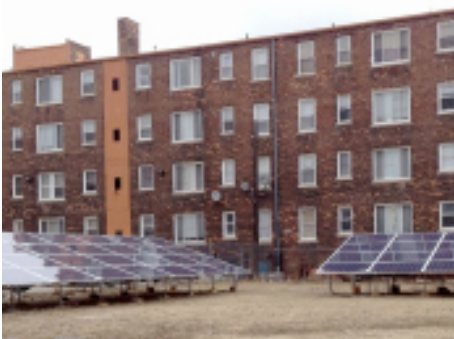
Figure 11: Multifamily apartment ground mount array in Detroit (Brainard St. Apts-Midtown)
