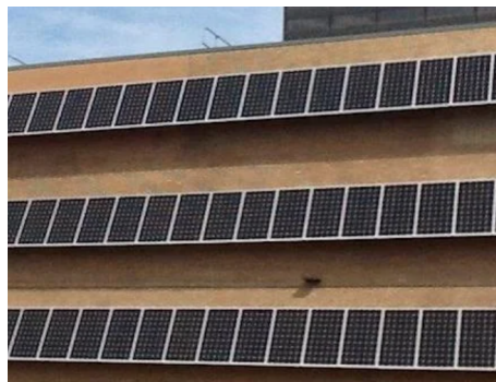
Figure 12: Commercial building with Building Integrated PV (BIPV) as facade - Detroit, MI (Navitas House-Downtown)
