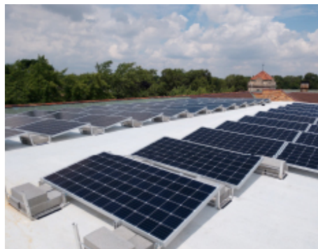
Figure 9: Gesu Catholic School rooftop array in Detroit (6 Mile-Northwest)
