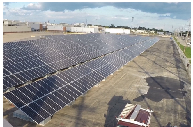
Solar array on GM Plant property in Warren, MI 6
