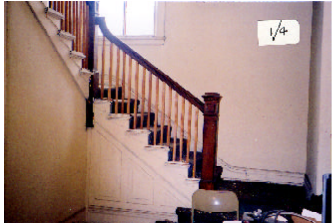
Stained Front Stair Railing
