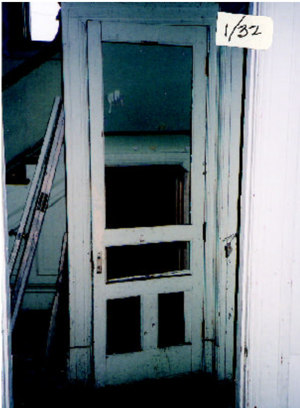
Damaged Five Panel Door (panels missing)
