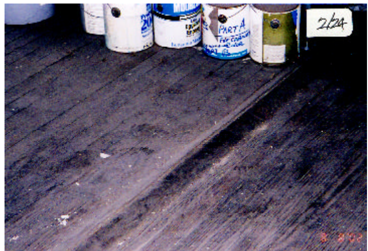
Wood Floor Needs Refinishing
