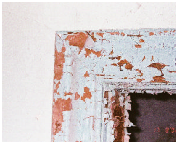
Damaged Paint Finish
