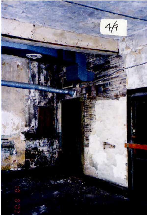
Deteriorated Plaster on Wood Lath
