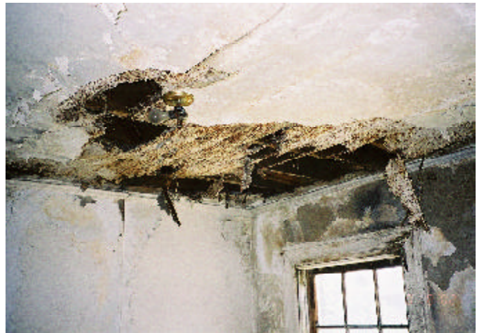
Extensive Deterioration and Collapse
