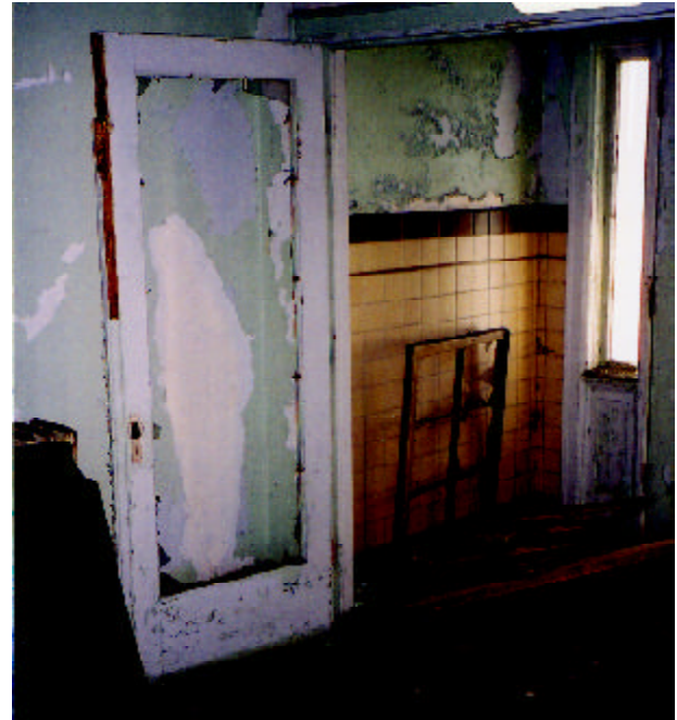
Damaged 15 Lite Glazed Door
