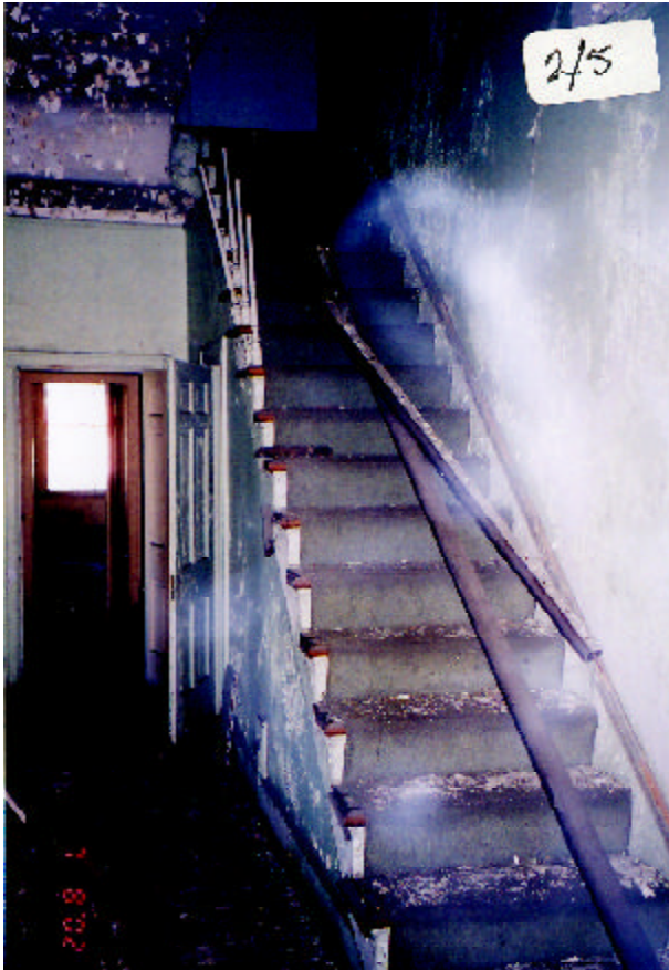
Entire Railing Missing
