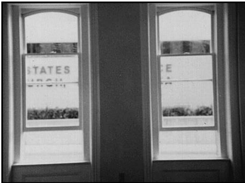
Figure 18.4 Deteriorated Window Sashes Were Replaced in This Historic Property While the Frames and Trim Were Wet Sanded and Repainted (vinyl liners were also installed as a friction reduction treatment).
