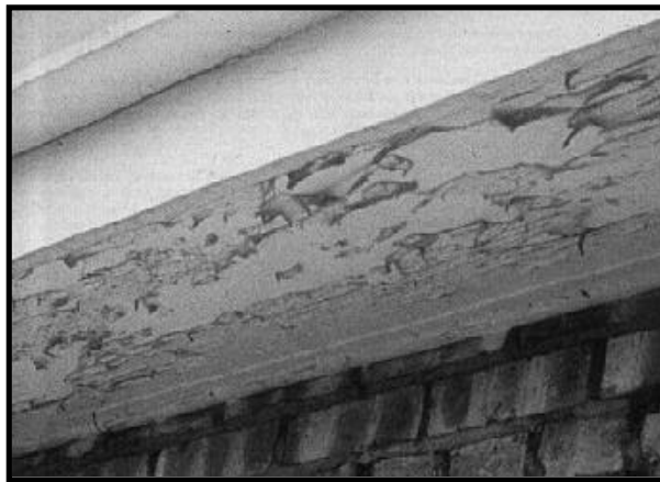
Figure 5.2b Forms of Paint Deterioration: Scaling, Cornflaking, and Peeling.
