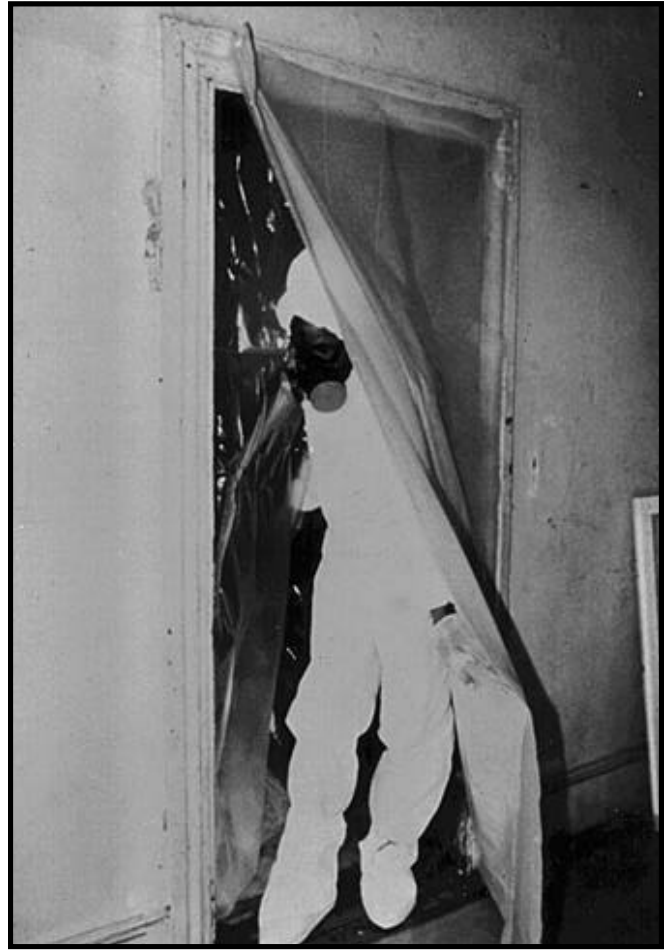
Figure 8.6 Install a Simple Airlock Over a Doorway to Minimize Lead Dust Migration.
