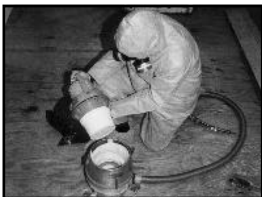
Figure 11.16e Wash or Replace Coarse Prefilters if Necessary.
