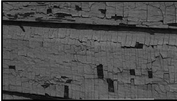
Figure 5.2d Forms of Paint Deterioration: Alligatoring.
