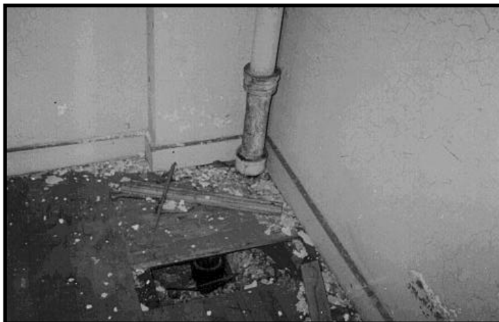
Figure 8.2 Area Should Be Precleaned and Structural Deficiencies in Flooring Repaired Before Lead Hazard Control Begins.
