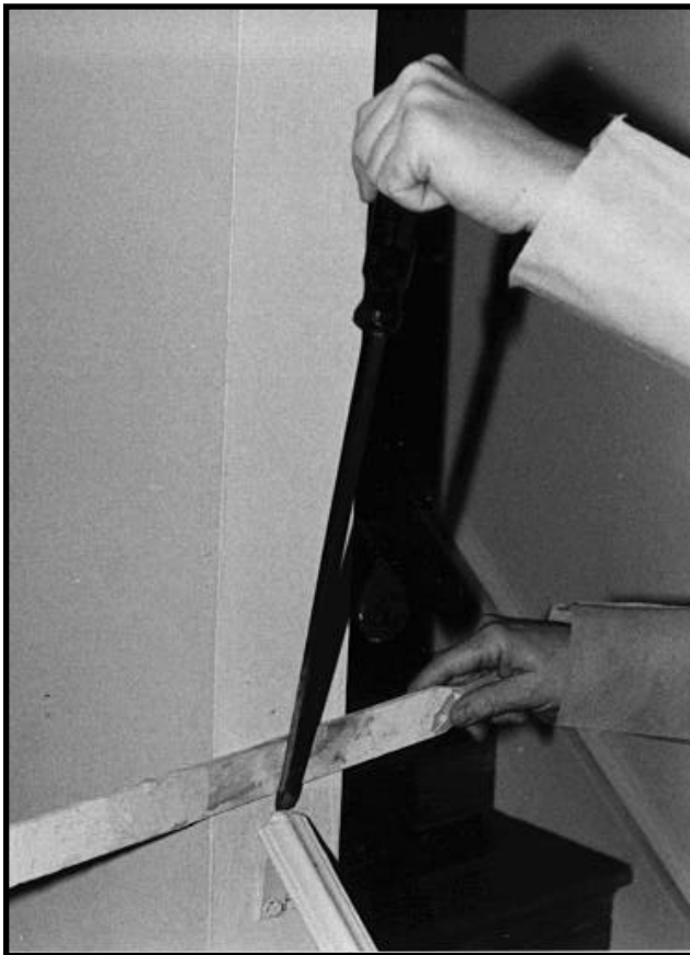
Figure 12.1 Use a Pry Point Pad To Minimize Damage to Adjoining Surfaces During Component Removal.
