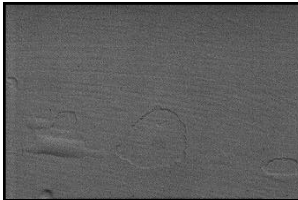
Figure 5.2e Forms of Paint Deterioration: Blistering.
