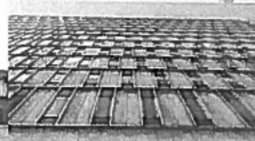
NATIONAL BANK OF DETROIT BUILDING RUNNING BOND MODULE OF WINDOWS AND MARBLE PANELS
