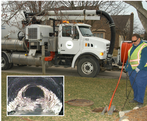
FOG build-up in sewer pipes (inset photo) requires local public works staff to go to the site and remove the blockage. The extra maintenance required to clean the sewer comes at a cost to all sewer system users.
