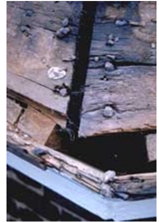
Analyzing the nail technology can help establish the period of construction and provide other important information. Photo: Travis C. McDonald, Jr.
