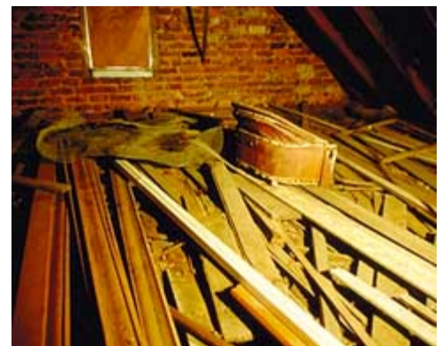
Discarded items are routinely stored within attics, then forgotten only to be discovered during a later investigation. Seemingly worthless debris may help answer many questions. Photo: Travis C. McDonald, Jr.
