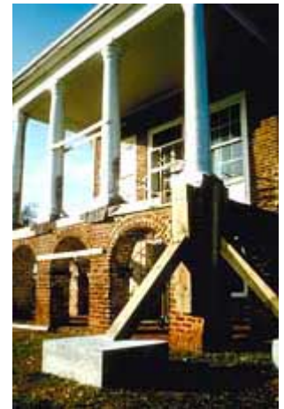
Investigation frequently identifies urgent needs of stabilization. Supplemental support, such as temporary shoring, may be required to prevent collapse. Photo: Travis C. McDonald, Jr.
