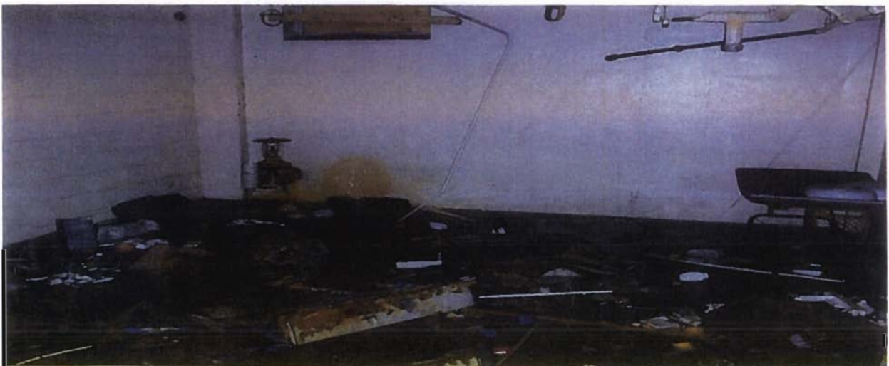
Vacant commercial property with running water creating soft soil outside the building, which could lead to structural problems.
