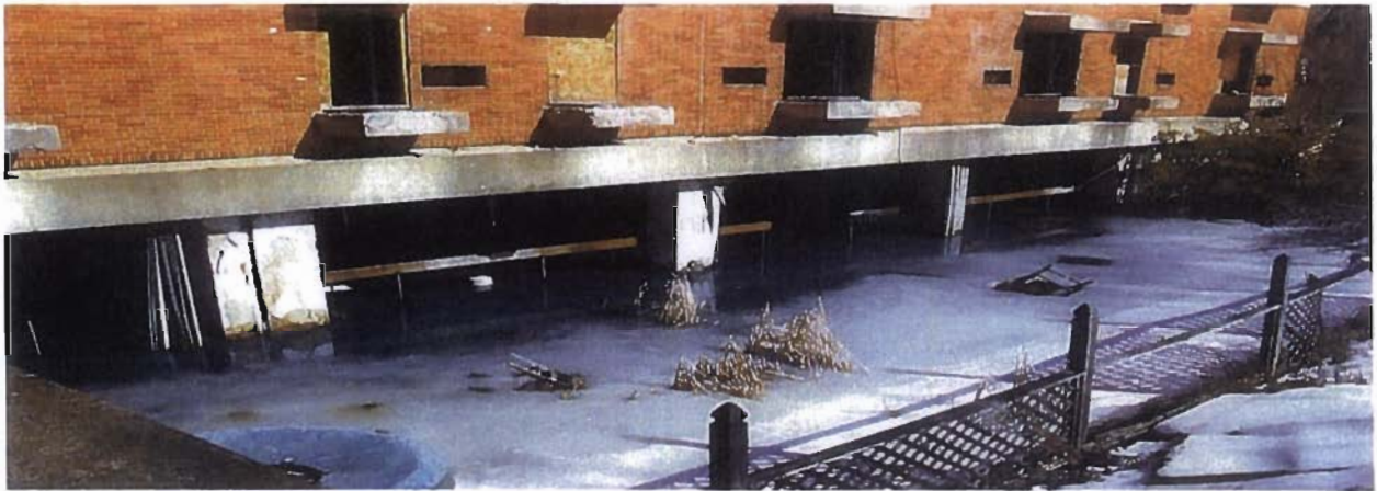
Vacant commercial property with six feet of water and mold.
