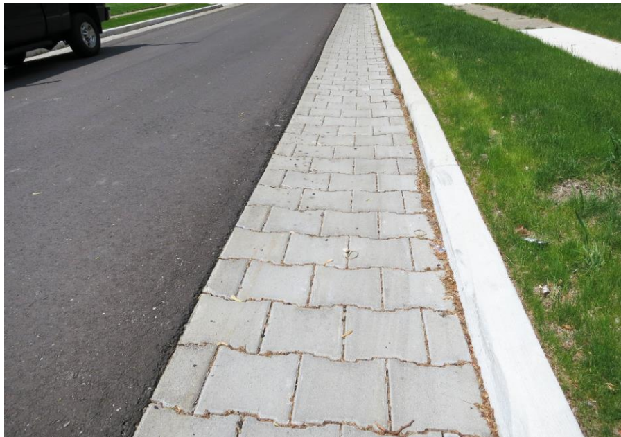
Figure 29 Keeler Street Permeable Pavers
