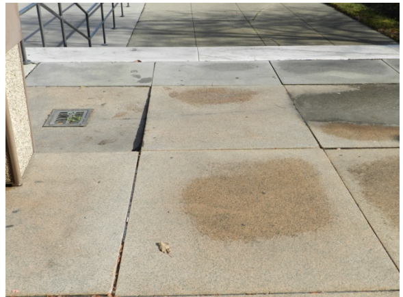
Main Library Woodward entry caving in
