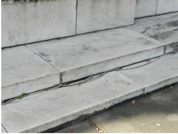
Main Library Woodward entry steps need repair
