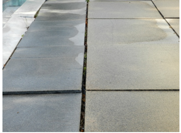
Main Library Cass Circle marble coming loose from the building
