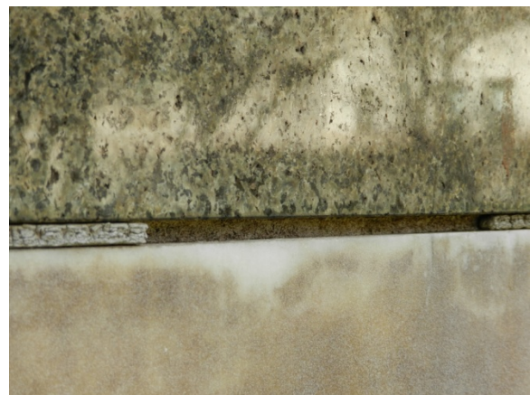
Main Library Eastwing sandstone needs cleaning
